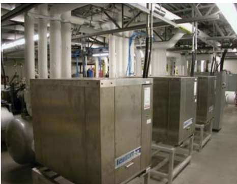
Central heat pumps
